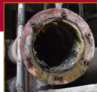
Metal pipe shown here exhibiting both internal and external corrosion.
