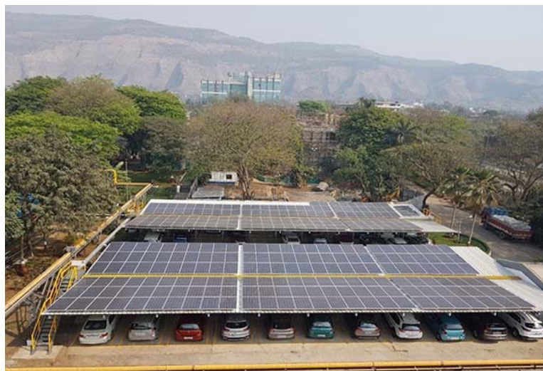
Solar panels at our facility in Mumbai, India.
